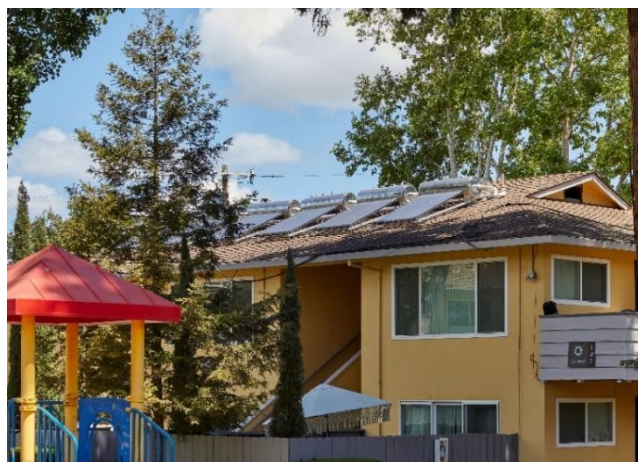
The new rooftop solar water heaters deliver hot water faster and improves the efficiency of the existing gas water heaters
